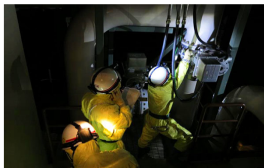
Drills opening valves used in containment vessel vents (Chubu Electric Power website)
